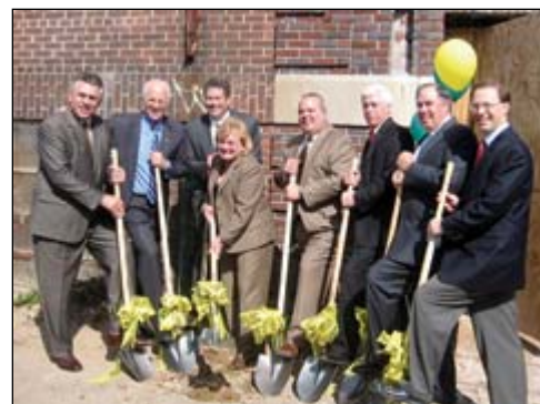
Groundbreaking at Olde School Commons, Bridgeport, Connecticut. Olde School is WNC's first property in Connecticut.
